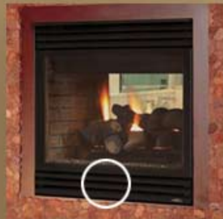
Behind the lower louvers
