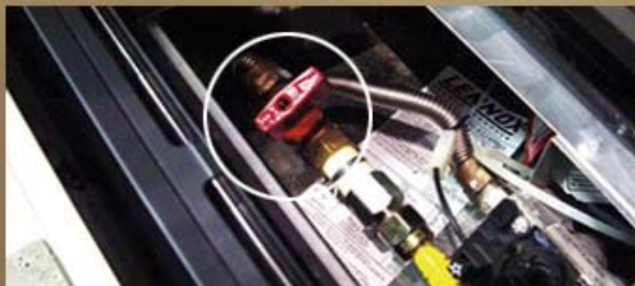
Gas supply in the OFF position
